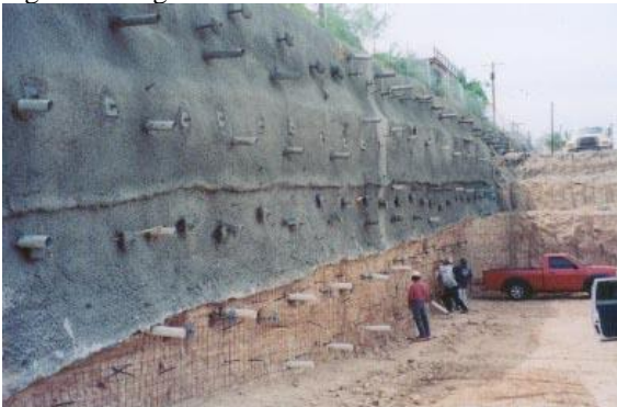
Photo 6-47 New retaining wall under construction using helical tension anchors as soil nails.
