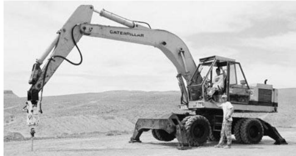
[Paper No. 2] Figure 2. Square Shaft Helical Pier Installation Using a Wheeled Hydraulic Excavator
