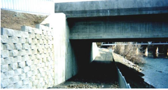
Photo 6-33 New reinforced concrete multi-lane bridge with abutments supported on helical piles and helical tiebacks.
