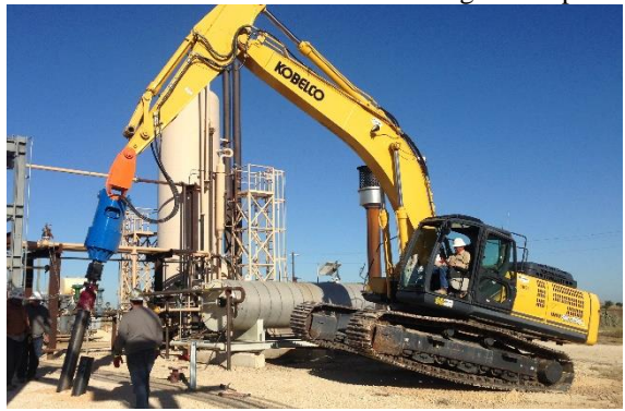
Photo 4-43 Large tracked hydraulic excavator installs large battered helical pile for high lateral load.
