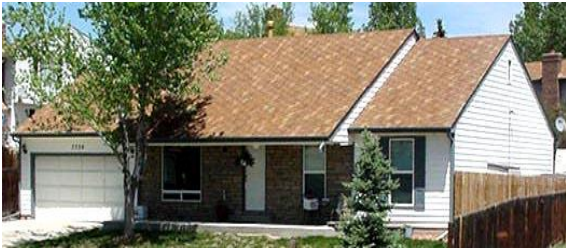
Photo 6-27 Existing residence with 18 inches differential heave in expansive soil underpinned, stabilized, and re-leveled on helical piles.
