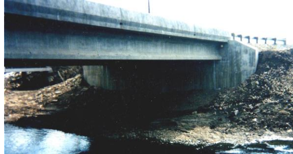
Photo 6-34 New reinforced concrete multi-lane bridge with abutments supported on helical piles and helical tiebacks.
