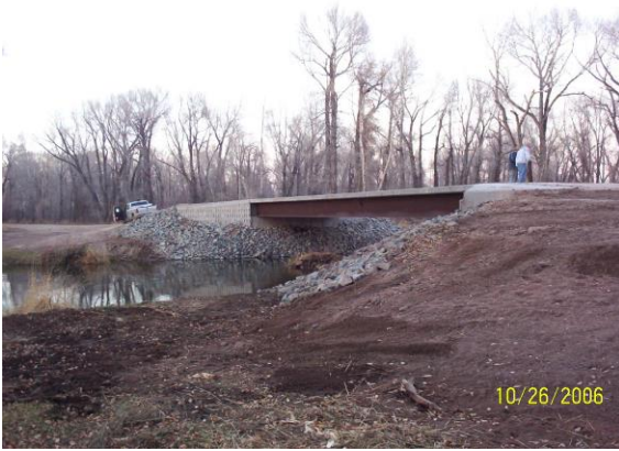
Photo 6-35 New steel bridge with abutments supported on helical piles and helical tiebacks.
