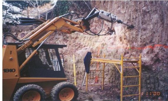
Photo 4-31 Skid-steer machine installing helical tension anchors as tiebacks for new retaining wall.
