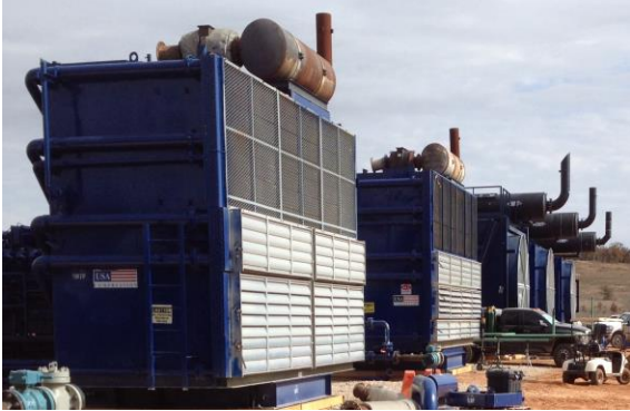
Photo 6-13 Compressors designed and constructed on helical piles with their high damping ratios.
