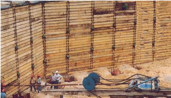
Photo 6-43 New soldier beam and wood lagging shoring wall using helical anchors as tiebacks.
