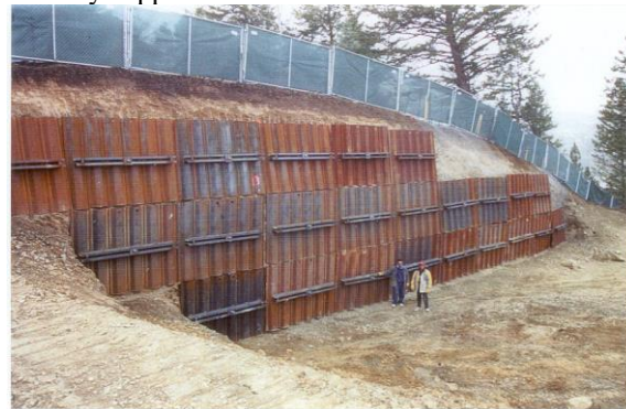
Photo 6-48 New pre-engineered shoring panel shoring wall using helical tension anchors as tiebacks.
