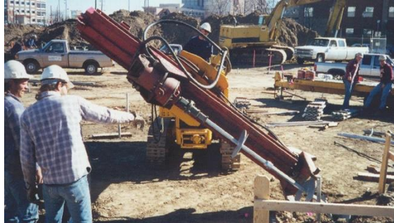
Photo 4-9 Tracked machine with adjustable frame installing battered helical piles for lateral loads.
