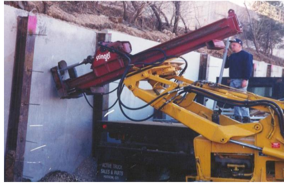
Photo 4-29 Loader mounted torque motor installing helical tension anchors as tiebacks for repair.
