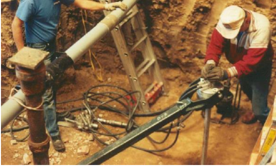
Photo 4-22 Hand-carried torque motor, yoke, and torque arm in tight access location.
