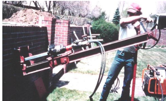
Photo 4-35 Hand-carried mast in near horizontal position installing helical tension anchors as tiebacks.
