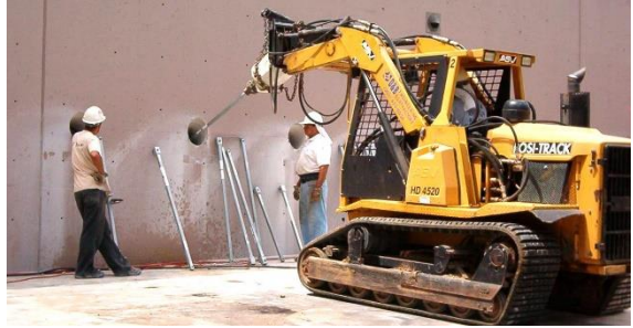
Photo 4-41 Tracked machine installing helical tension anchors as tiebacks for retaining wall repair.
