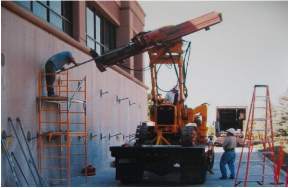
Photo 4-28 Tracked machine to install helical tension anchors as tiebacks for retaining wall repair.
