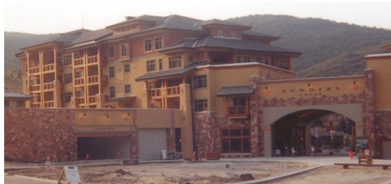
Photo 6-32 Existing building still under construction settled. Foundation underpinned and stabilized with helical piles.
