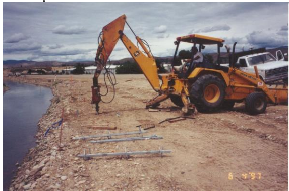
Photo 4-39 Backhoe installing helical screw piles at a slight batter for a sound wall.
