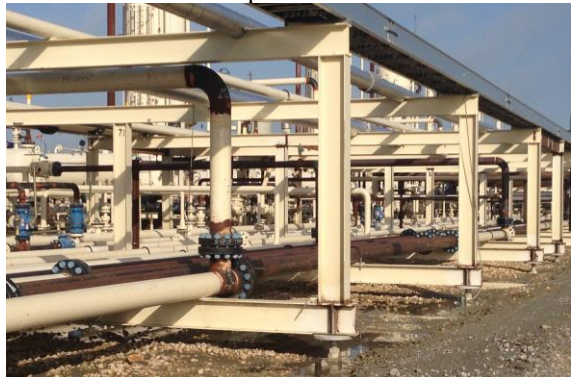
Photo 6-12 Pipe rack with high lateral loads and moments designed and constructed on helical piles.
