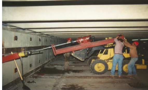
Photo 4-33 Skid-steer mounted drive head installing helical tension anchors as tiebacks in low overhead.
