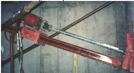
Photo 4-50 Hand-carried mast mounted on wall in near horizontal position to install helical tiebacks.
