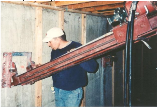
Photo 4-26 Hand-carried mast in near horizontal position to install helical tiebacks in low overhead.
