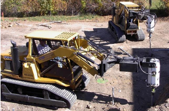
Photo 4-8 Two tracked machines each capable of installing over 60 helical piles per day.
