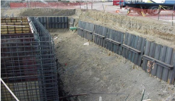
Photo 6-45 New pre-engineered shoring panel shoring wall using helical tension anchors as tiebacks.
