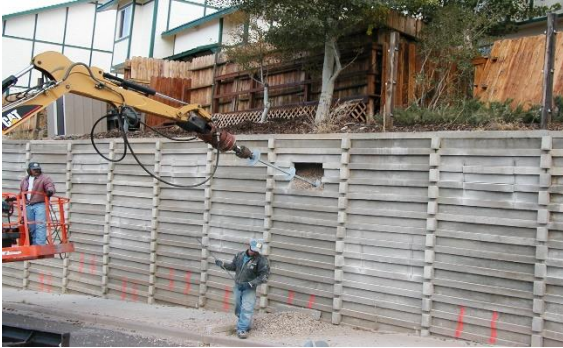
Photo 4-32 Backhoe mounted torque motor installing helical tension anchors as tiebacks for repair.
