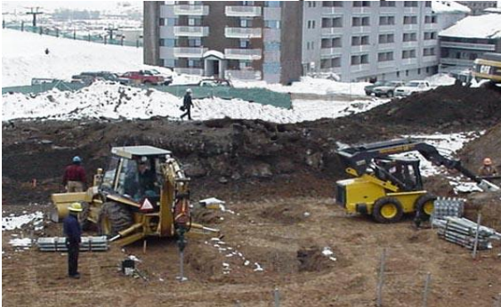
Photo 4-30 Skid-steer machine (on right) installing helical tension anchors as tiebacks for structure.
